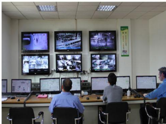
▲ Master control room
